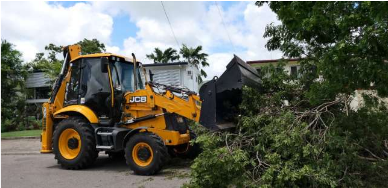
Council crews were deployed across Townsville to clean-up hazardous green waste following Tropical Cyclone Kirrily.
